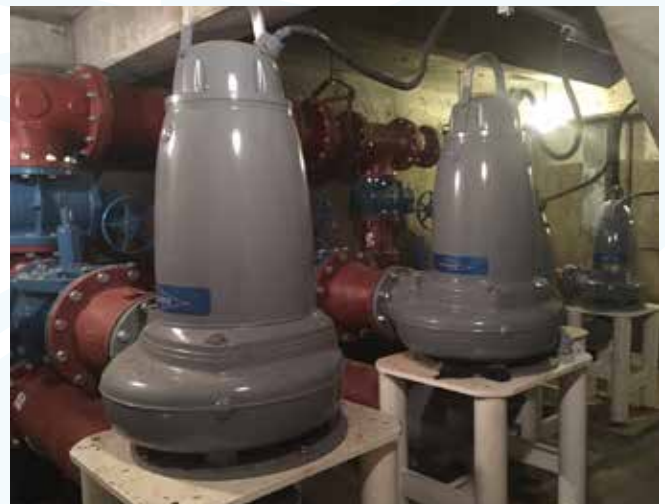
Triplex head works pump station upgrade.
